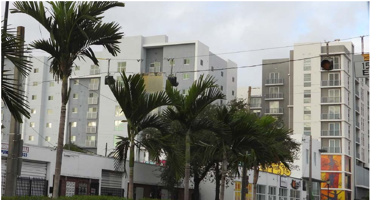
General Photographs. East Elevation. Visible stains and cracks.
