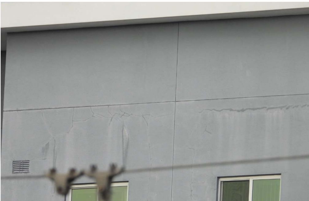
East Elevation. Typical. Visible stains and cracks along the unaddressed slab deflection joints and additional cracks propagating from corners of openings. Also visible efflorescence.
