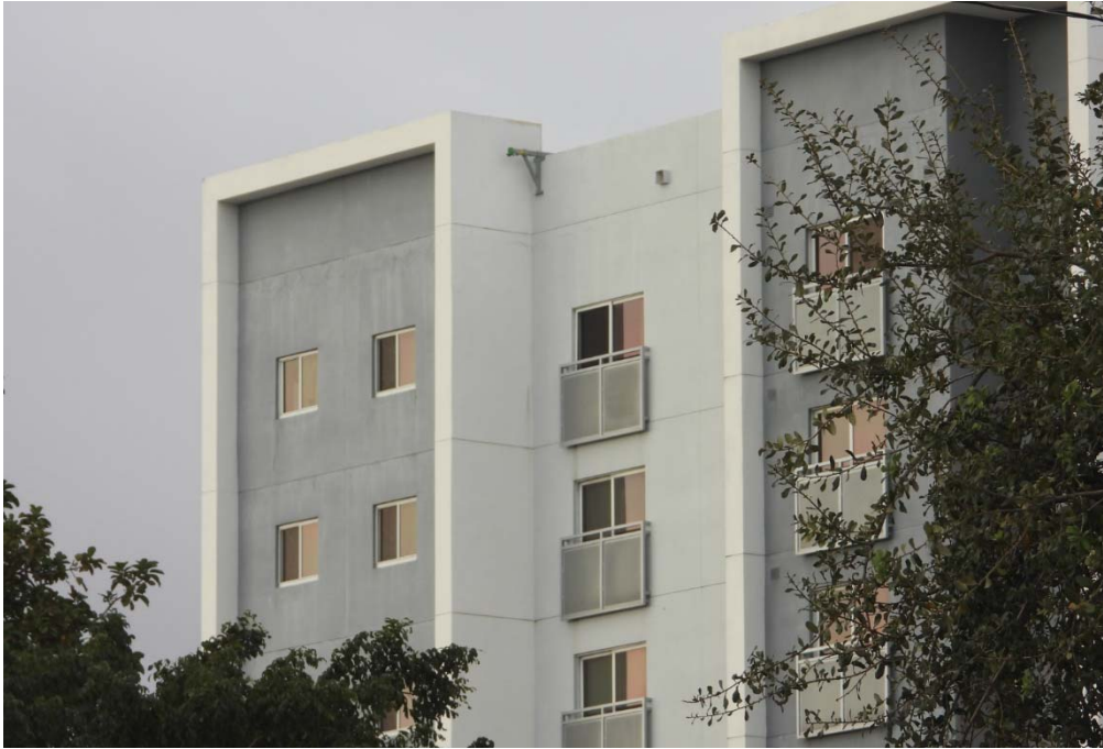
East Elevation. Typical. Visible stains and cracks along the unaddressed slab deflection joints and additional cracks propagating from corners of openings. Also visible efflorescence.
